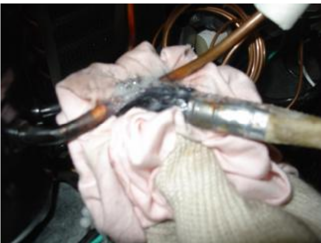
j. Connect the vacuum pump with the processing tube and then vacuimize for more than 20 minutes.
